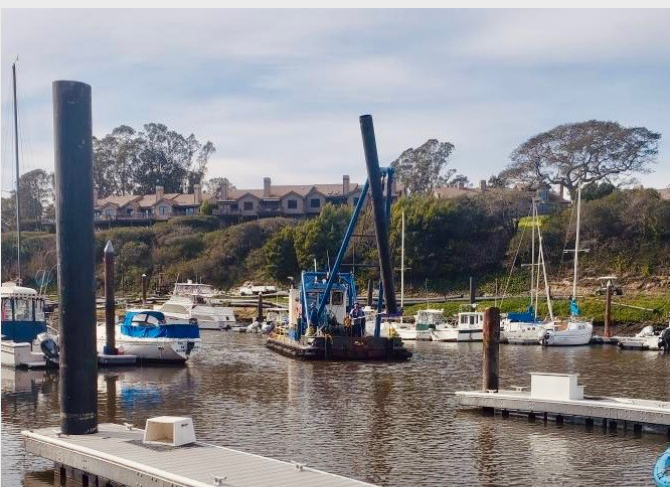
Pictured above, maintenance and dredge crews utilizing the District's workboat, Dauntless , to repair one of the broken pilings on January 18, 2023.
