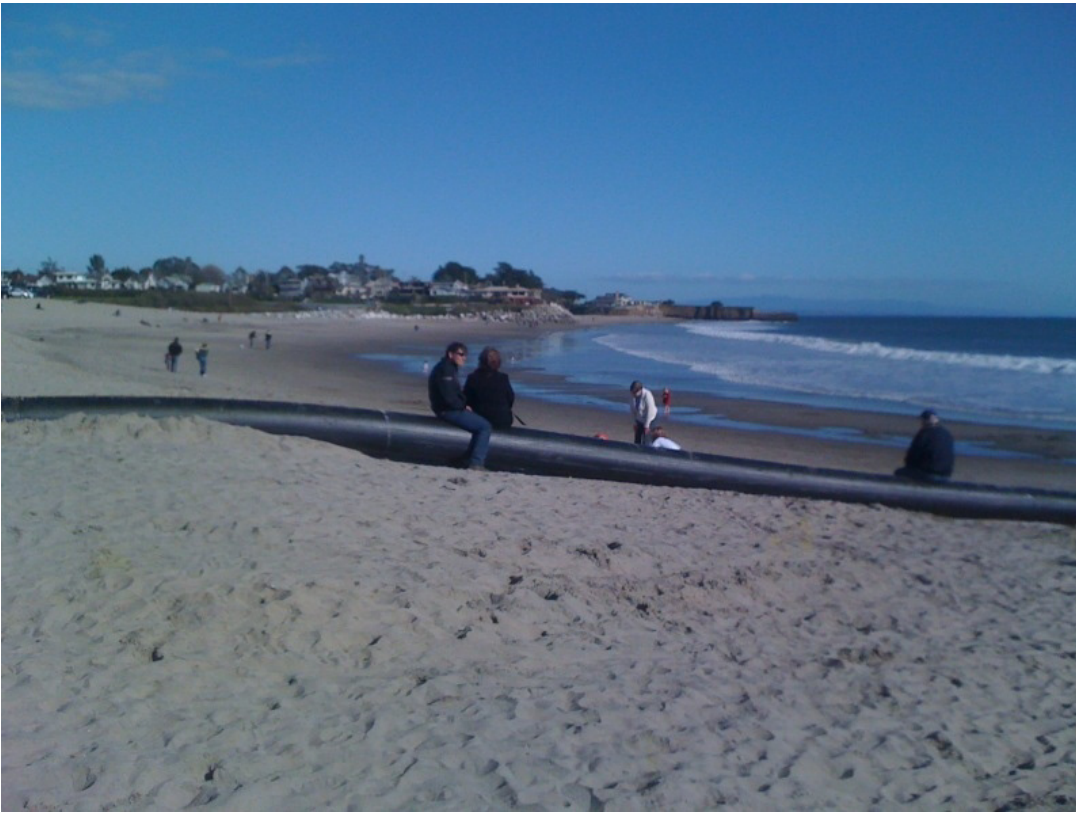
5. Pipeline on Beach
