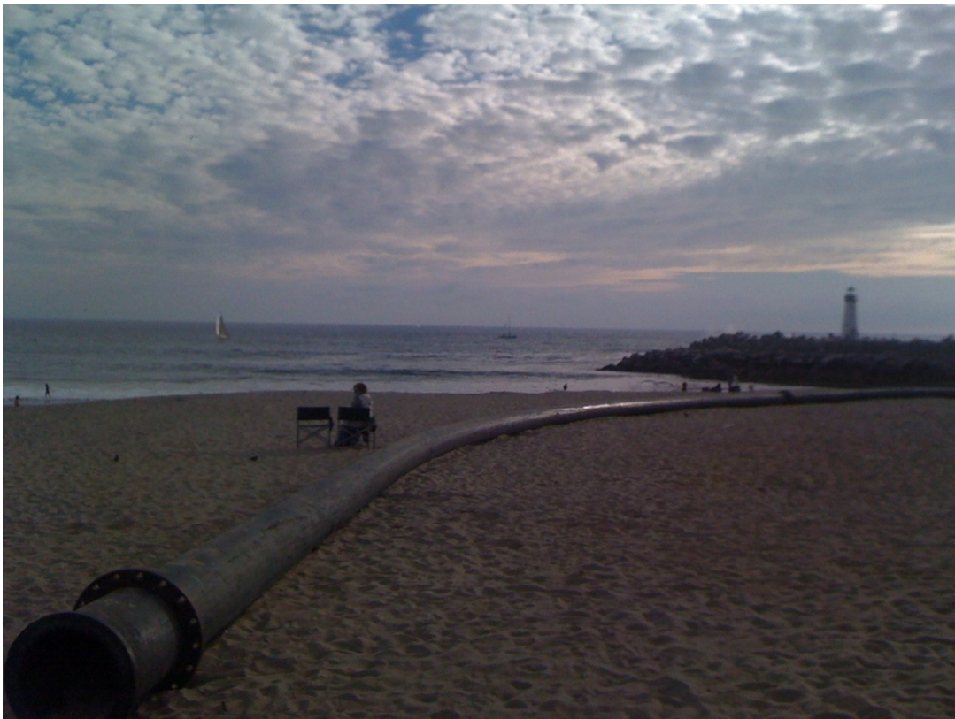
6. Pipeline on Beach
